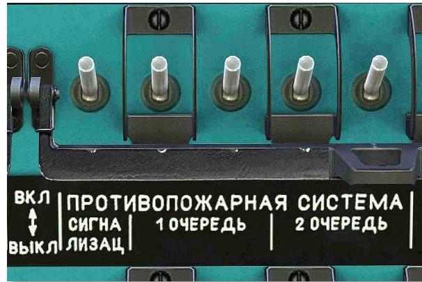
Fig. 7.25. Fire Protection System circuit breakers
